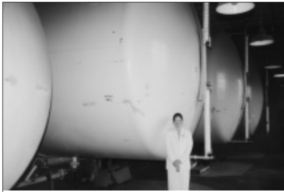
Liquid waste holding tanks in NADC's waste treatment plant, one of the Utility Buildings built in 1961.
